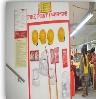
Fire Fighting Equipment
