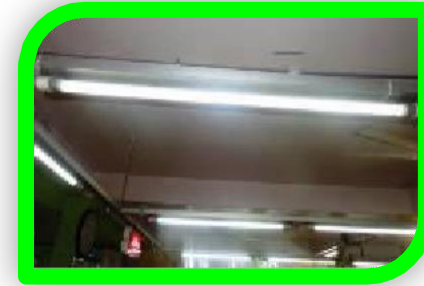
Energy Efficient Lighting
